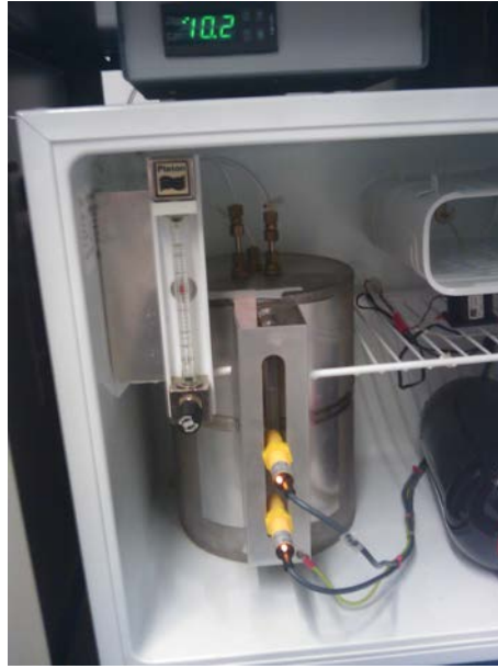
Fig. III.5: Photograph of the cupboard located underneath the quadHIDAC. It contains a fridge with a vapor used for the gas supply and the high voltage power supplies (not shown here) [Bol10].
